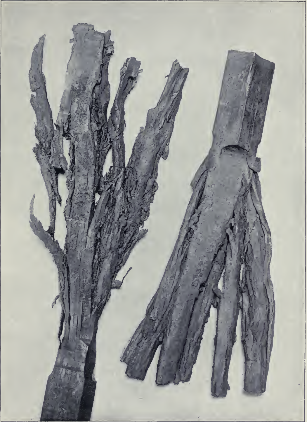
FIG. 62. DISINTEGRATED WROUGHT-IRON BARS
